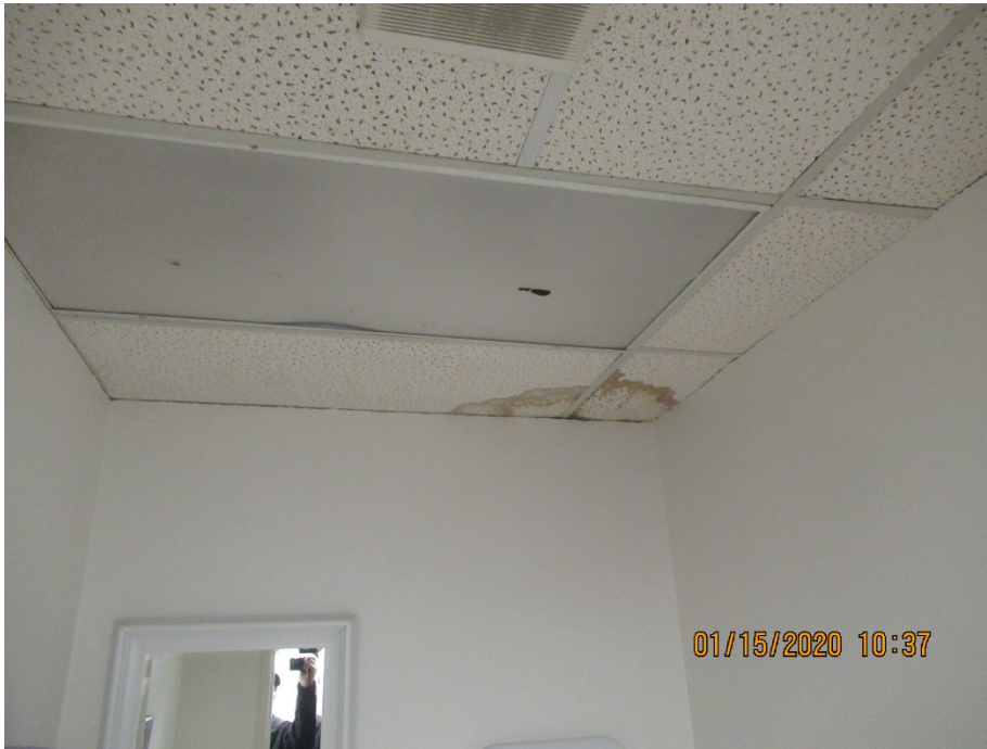
19. Water-stained ceiling tiles.
